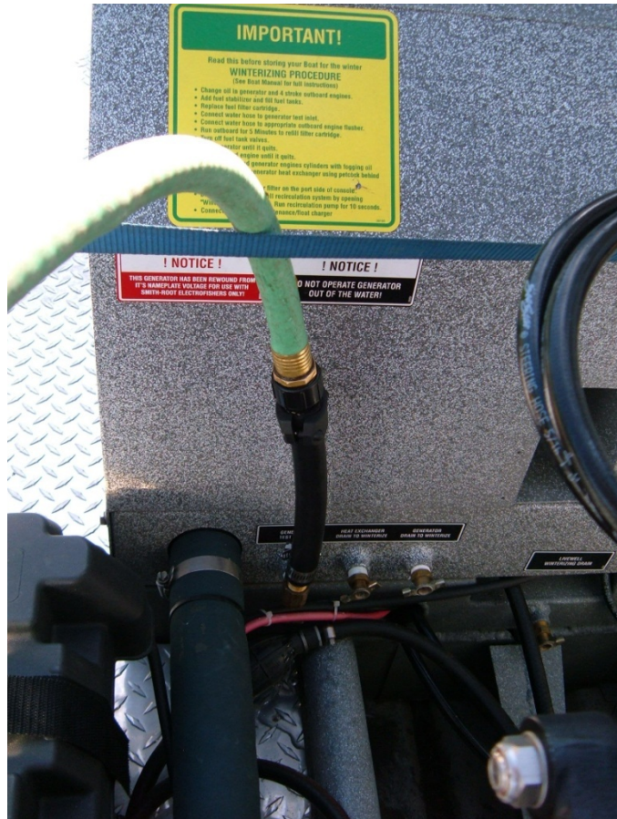
3C. Pipe plug has been removed, and generator flushing adapter has been attached.
