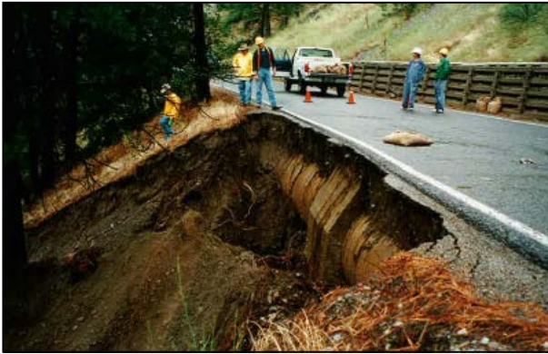
FIGURE 2-1 1996 Image of a Near-Failure of the Interceptor along Aubrey L. White Parkway
