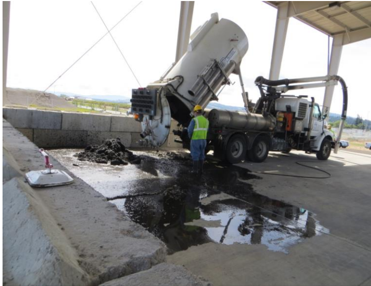
Fig-1 City of Spokane Decant Facility – vacor unloading
